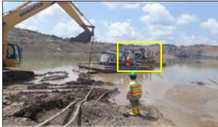
Gambar 4.3 Pompa Inveco 350 KW
